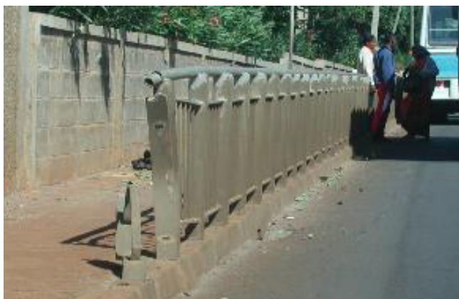
Figure 4.10: Poorly maintained pedestrian guardrail—Maintenance Inspection.
