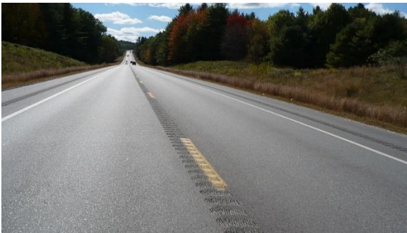
Figure 2. Centerline rumble strips provide tactile feedback to deter unintentional crossing of the centerline (Massachusetts, USA). Photo: SayCheeeeeese/Wikimedia Commons
