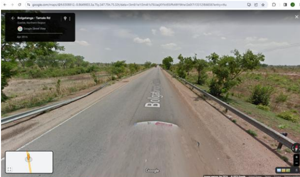
Figure 8. Damaged guard rail (northern Ghana 2016) Source: Google StreetView.
